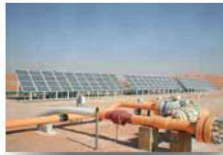
2004 - ALGERIA CATHODIC PROTECTION
